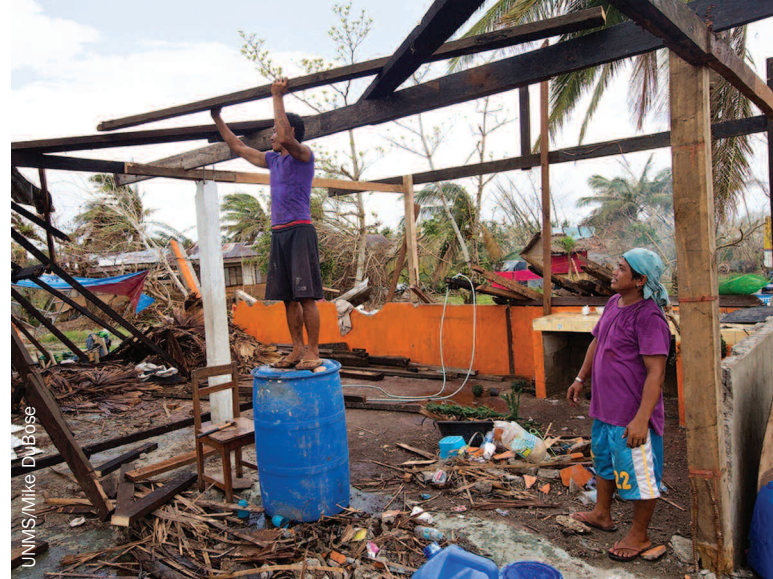
Neighbors work to erect a temporary roof on a home that was laid open to the sky by Typhoon Haiyan in Tacloban, Philippines. The powerful storm destroyed 1 million homes and displaced more than 4 million people. IOCC is responding with building materials to help families repair homes & construct temporary shelter in the country's hardest hit areas.
